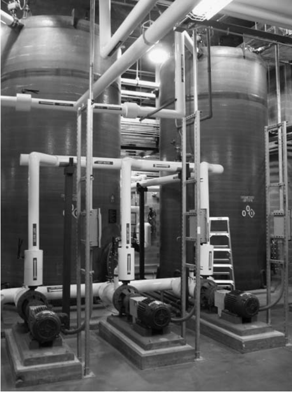
FIGURE 7 High-capacity soft-water storage and distribution: 304L stainless steel piping, fiberglass reinforced plastic (FRP) storage tanks, insulated for sweat control, and installed spare pump. Source: Courtesy of Lonza Biologics, Portsmouth, New Hampshire, U.S.A.
