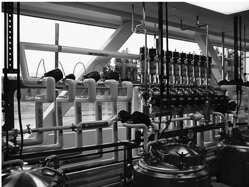
FIGURE 9 Photo of actual CIP supply loop and distribution valves for the process of Figures 5 and 8.
