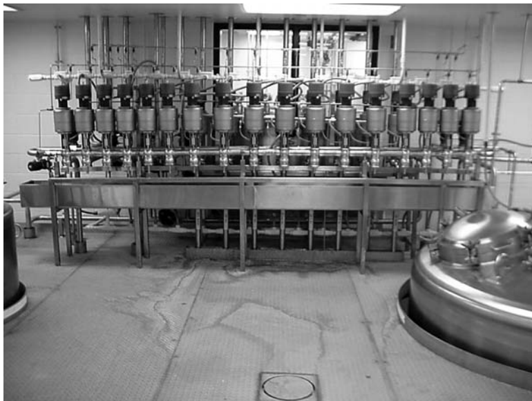
FIGURE 6 This mixproof valve manifold interfaced three Media Prep vessels to 10 hold tanks to support four chromatography columns in a highly automated CIPable process.
