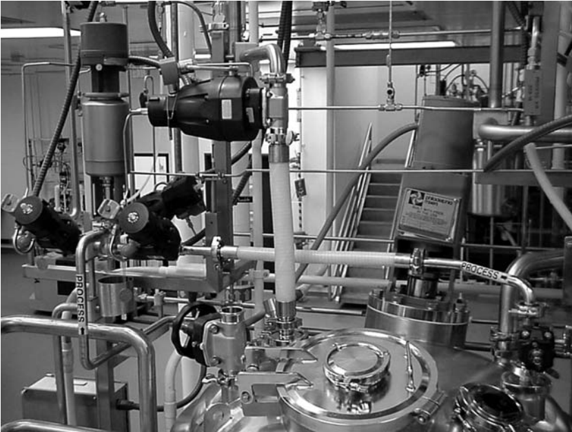
FIGURE 16 This tank top photograph shows the application of a rising stem mixproof valve in combination with diaphragm valves as shown schematically in Figures 9 and 15.
