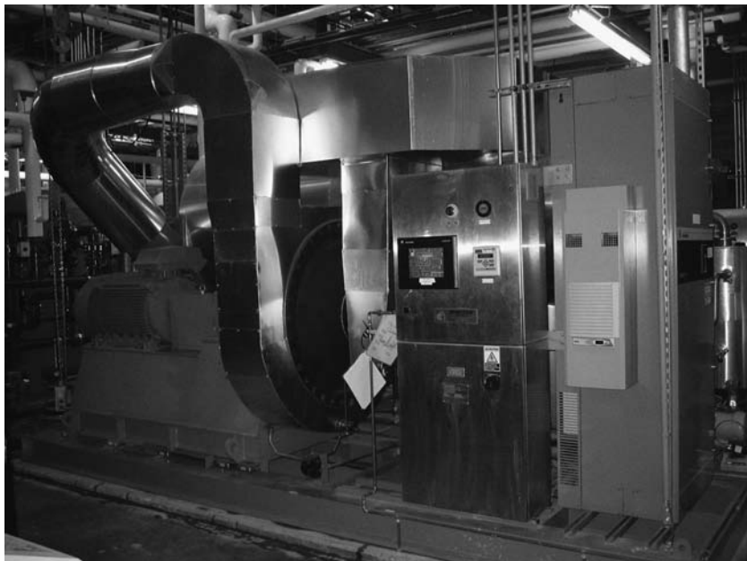
FIGURE 3 Vapor compression water-for-injection (WFI) still. Source: Courtesy of Lonza Biologics, Portsmouth, New Hampshire, U.S.A.
