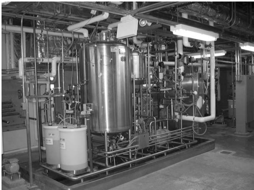
FIGURE 1 CIP skid in stainless steel containment pan. Source: Courtesy of Lonza Biologics, Portsmouth, New Hampshire, U.S.A.
