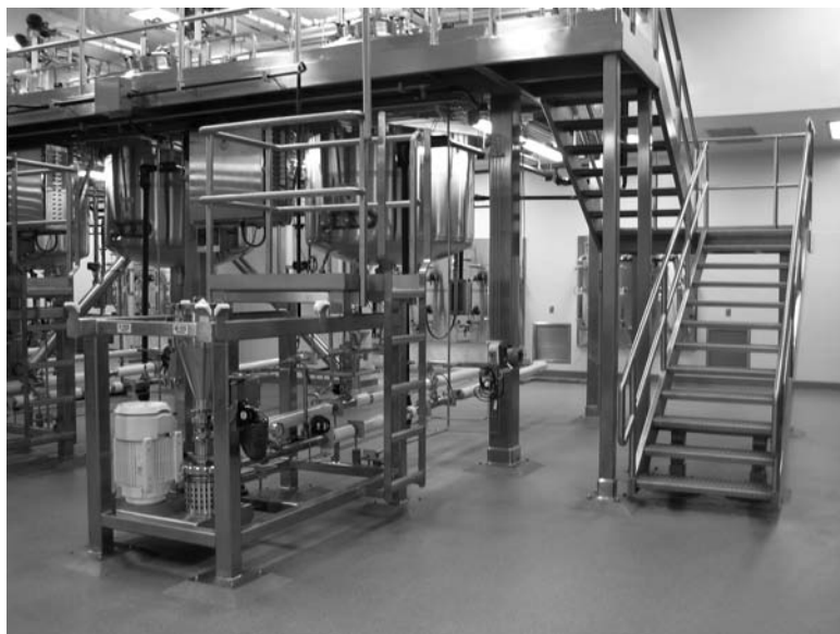
FIGURE 13 This photograph shows a high-capacity dry powder blending system in the outlet leg of a buffer prep vessel. The blender pump serves also as the filter supply pump and CIP return pump.
