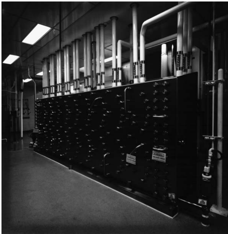
FIGURE 2 This larger process/clean-in-place transfer panel utilized loop-type headers and two different U-Bend lengths to configure a product development suite for a multiplicity of operations, all fully automated. Source: Courtesy of Electrol Specialties Company.
