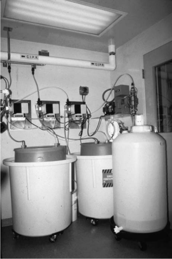
FIGURE 4 Electromagnetic-operated diaphragm pumps (three smaller pumps on left), a motor-operated diaphragm pump (larger pump on right), and portable secondary containment dollies for chemical drum handling.
