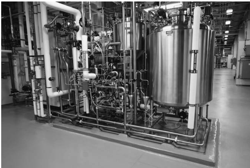
FIGURE 7 Eductor-assisted CIP skid with single water-for-injection tank located within a curbed area to confine minor leakage. Access for maintenance is excellent. Source: Courtesy of Genentech, Inc.
