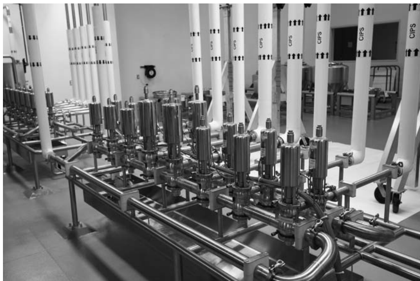
FIGURE 4 A rising stem mix proof valve array used to control clean-in-place (CIP) supply distribution from two CIP skids to eight circuits. A similar valve array in the left background controls return flow. Source: Courtesy of Genentech, Inc.
