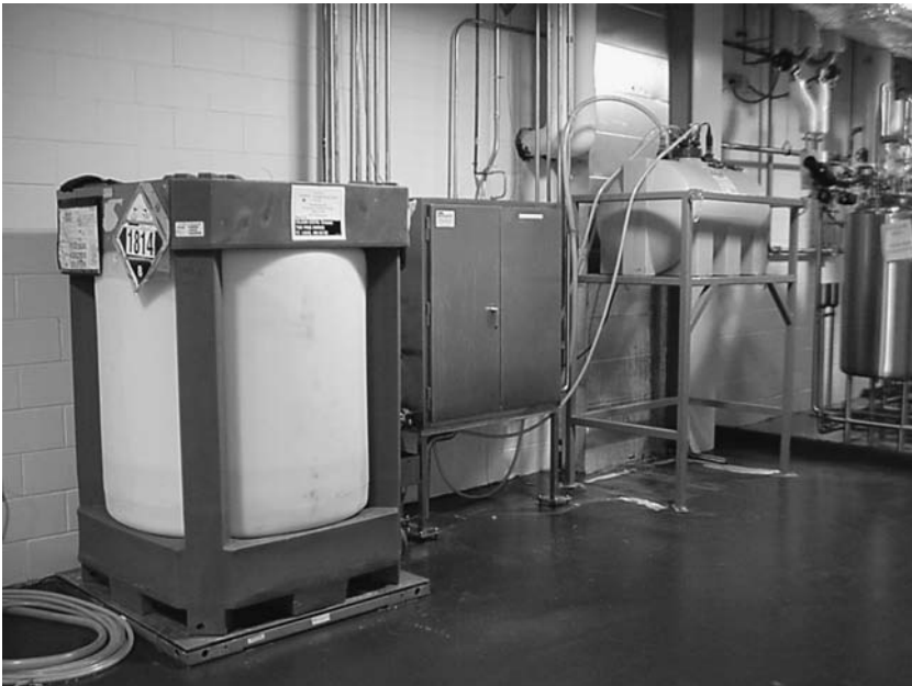
FIGURE 3 A bulk detergent tote on the left, day-use tank container on the right, and a stainless steel chemical feed pump enclosure supports multiple CIP skids.
