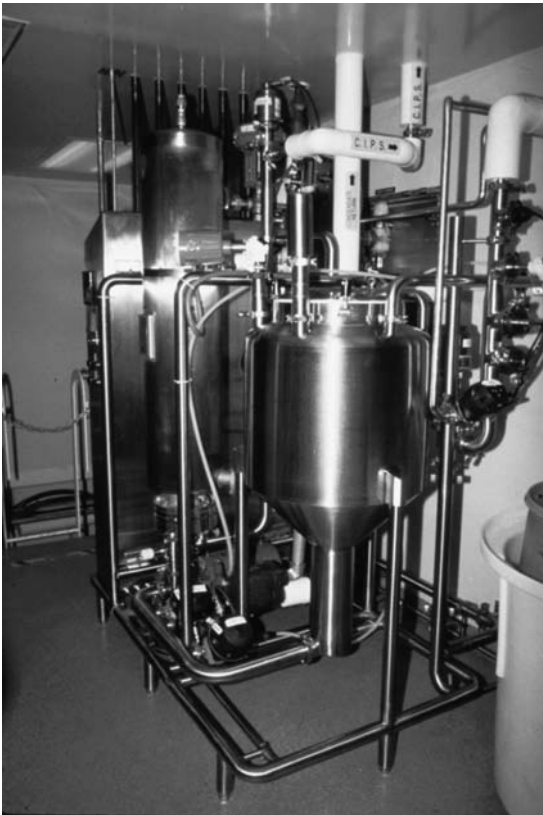
FIGURE 5 This total recycle clean-in-place skid can operate at up to 80 gal/min with an adequate water supply, and occupies an area of only 36 in. by 84 in., including the control panel.
