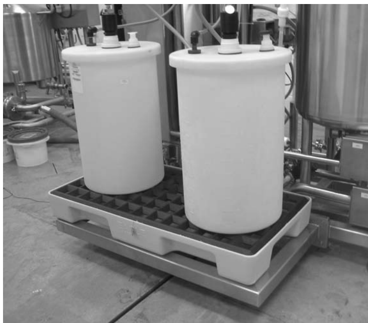
FIGURE 1 A commercially available spill pallet containment system installed as part of a prefabricated modular CIP system.
