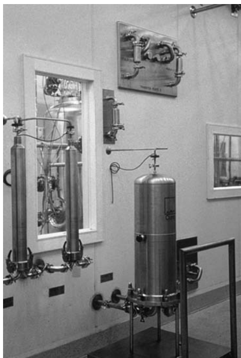
FIGURE 5 This view of a 1982 vintage sterile process shows U-Bend TPs installed through the wall between the clean room and the gray space in which the vessels and piping are located. Note use of TPs to mount filter housings. Abbreviation: TP, transfer panel.
