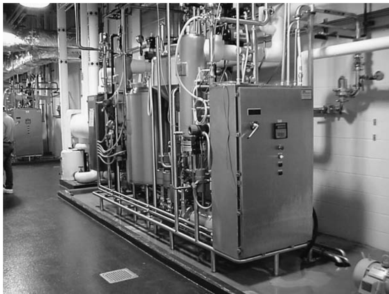
FIGURE 14 This single-use eductor-assisted CIP skid has a second CIP pump and heat exchanger on the left-hand end as a system capable of supplying flush, wash, and rinse solutions to a ultrafiltration process skid, from a common water tank.
