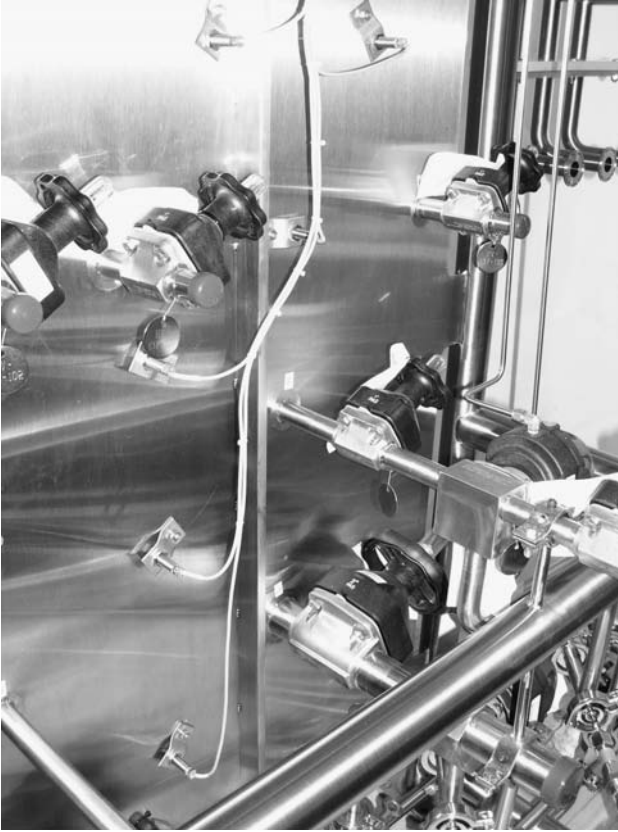
FIGURE 8 Transfer panel with U-Bend monitoring proximity switches.
