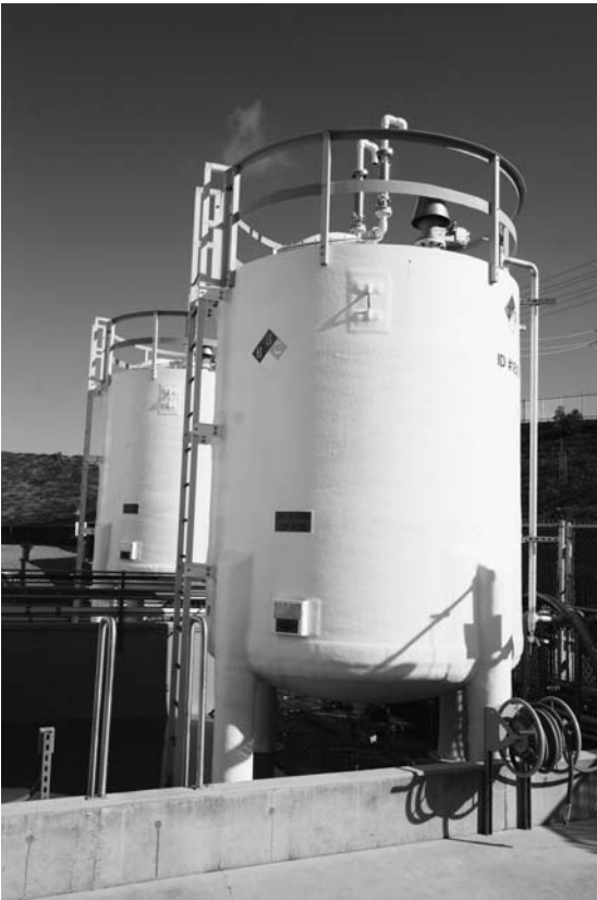
FIGURE 5 Externally mounted bulk storage tanks for caustic and phosphoric acid cleaning chemicals handled by bulk delivery and storage. Distribution to the individual CIP skids was by chemical headers, valves, and magnetic flow meters. Source: Courtesy of Genentech, Inc.
