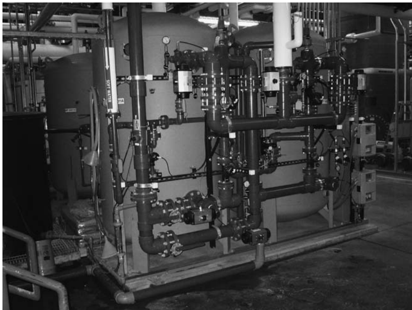
FIGURE 2 Dual water softener system. Source: Courtesy of Lonza Biologics, Portsmouth, New Hampshire, U.S.A.
