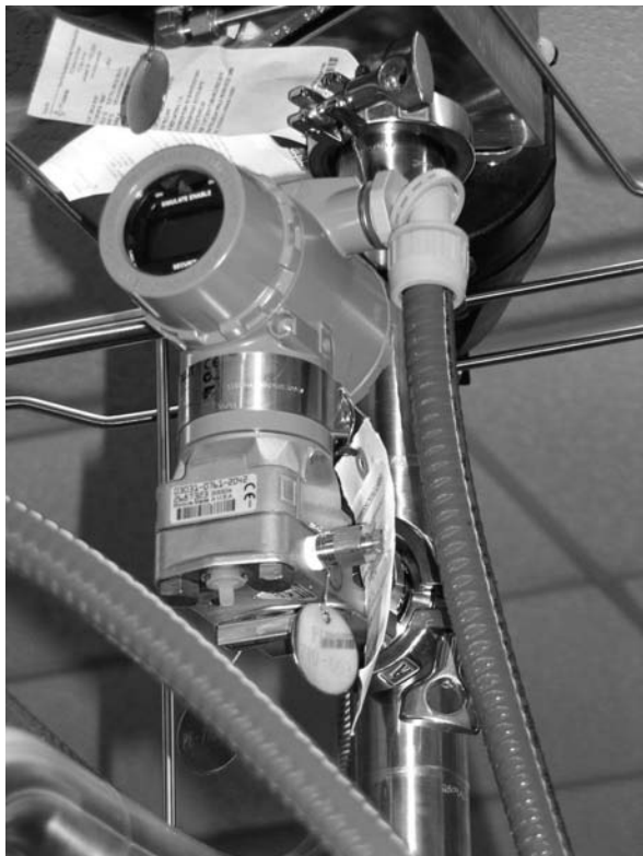
FIGURE 16 Pressure sensor with nonmetallic conduit.
